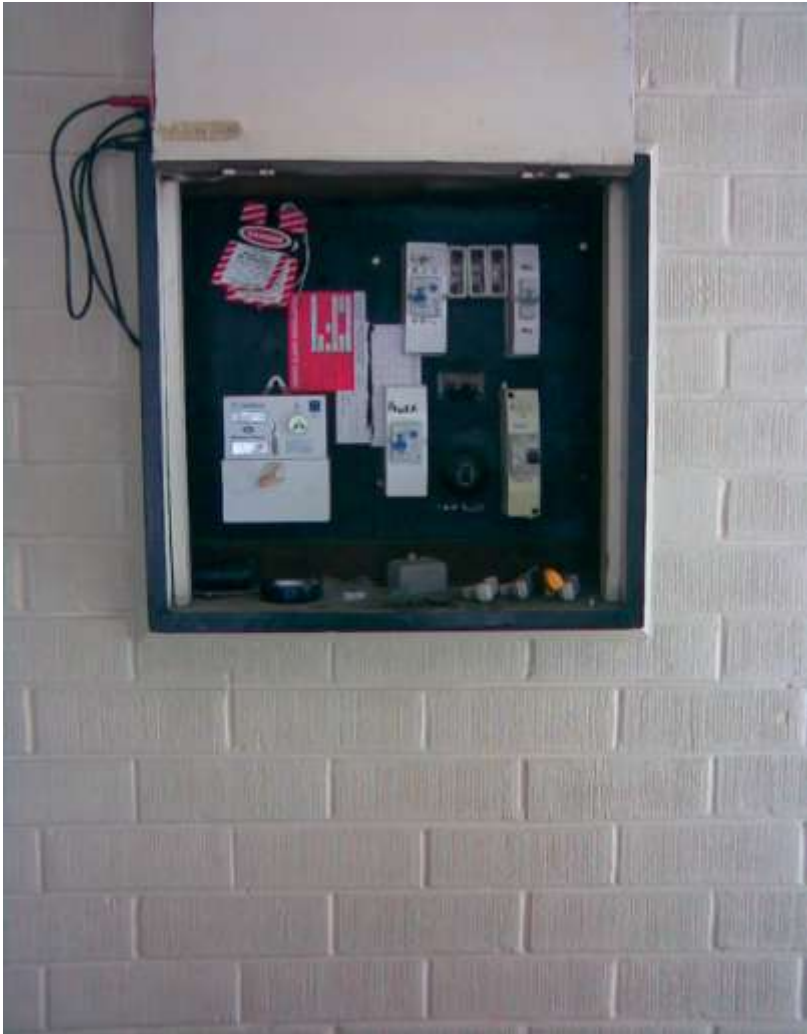
Isolation of circuits at fuse board
