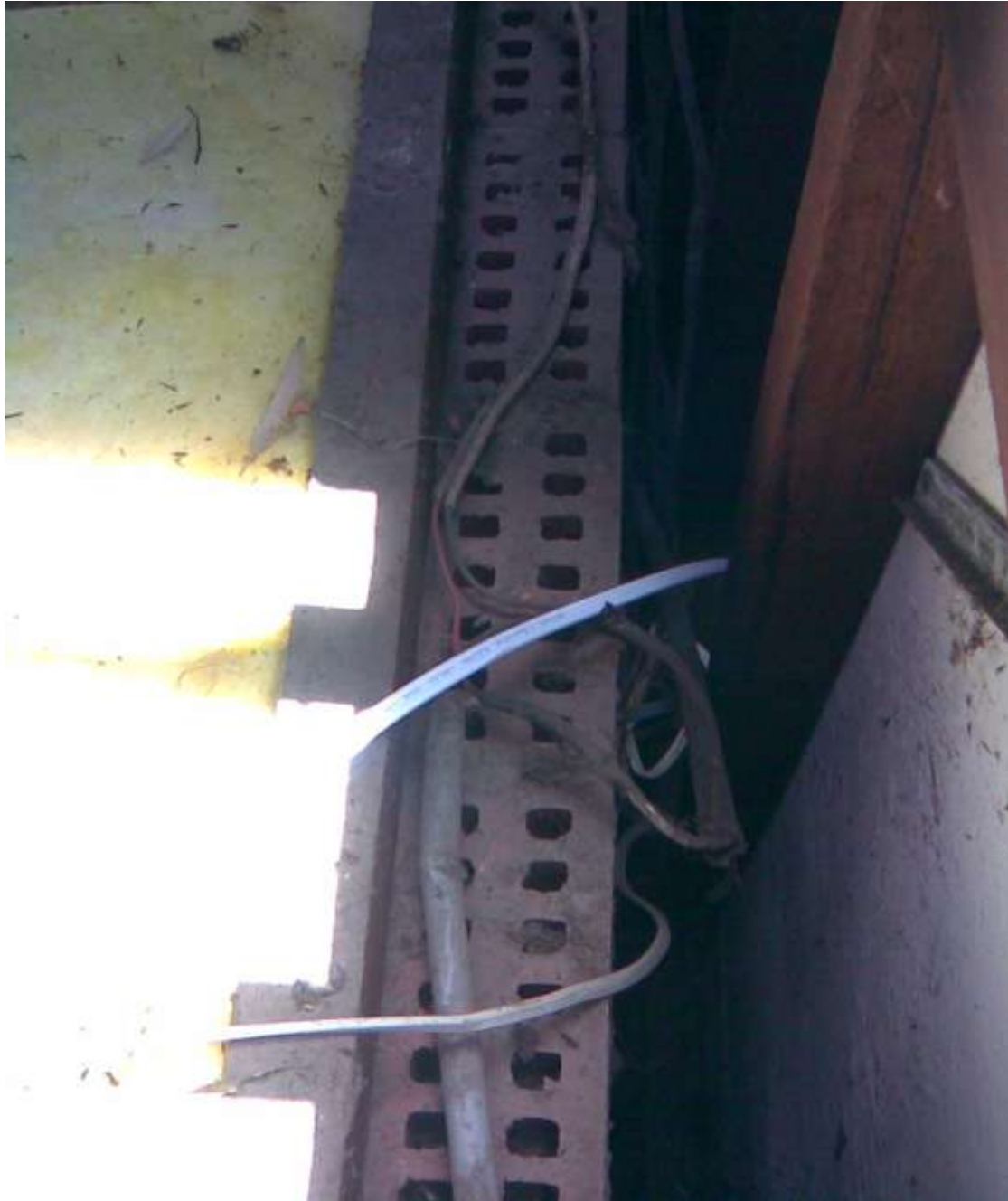
Location in roof space where the incoming main cables were spliced into, note in order for this to have occurred the connection would have had to be carried out live!
